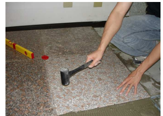
insert tile spacers, form 2 mm gap for grouting, check leveling in sequence
